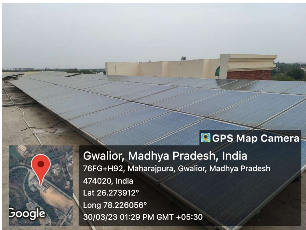
Solar Power Plant
